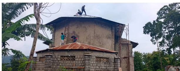
Workers repair the choir roof. The lower area with the rusty roof is the Sacristy.
